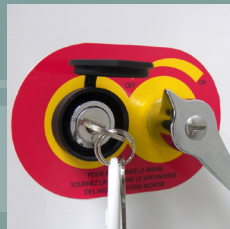
Secured disinfection valve
